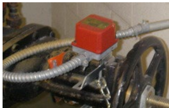
Tamper switch on a sprinkler valve
