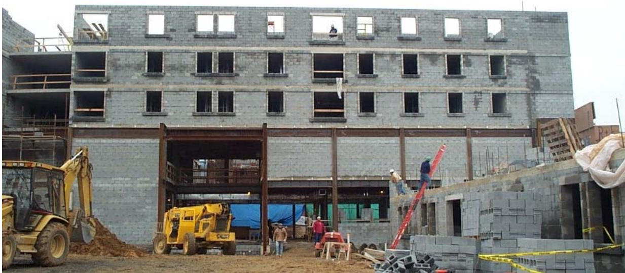
Figure 5: Building C – The steel frame on the first two floors coupled with load bearing masonry walls on the upper floors can be seen.
